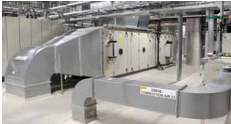
The new DAF Engine Test Center – which has created about 80 additional, skilled jobs – has three storeys. The basement contains technical installations. The test cells and inspection areas are on the ground floor, whilst the first floor is fully occupied by equipment for air and water treatment. Each hour these facilities are able to recirculate 36,000 m 3 of air per test cell, to cool the engines with water, to feed conditioned combustion air and to transport away monitored – noise-damped – exhaust gases.
